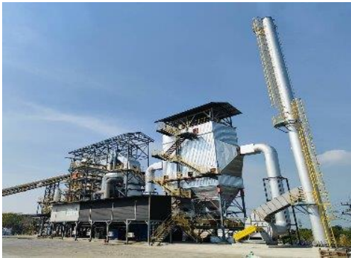
Reduce natural gas usage by utilizing Biomass boiler
